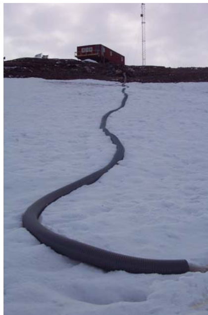
Figure 12: Wastewater pipeline at Wasa station Source: Swedish Polar Research Secretariat
